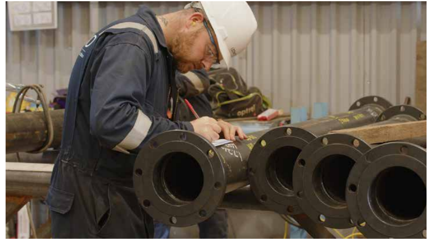
Photo courtesy of Ledwood Mechanical Engineering.
